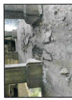
① : Spall Repair on South Arch. (South Arch Shown, North Arch similar)
