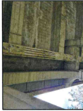
16 : Spall Repair on Span 14 Exterior Girder. (North Girder Shown, South Girder Similar)
