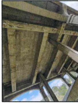
15 : Spall Repair on Span 13 Exterior Girder. (South Girder Shown)
