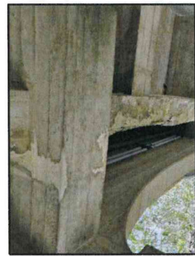
⑥ : Spall Repair on Span 4 exterior Girder. (South Girder Shown, North Girder similar)
