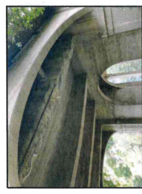
①: Spall Repair on exterior Girder. (South Girder Shown, North Girder similar)
