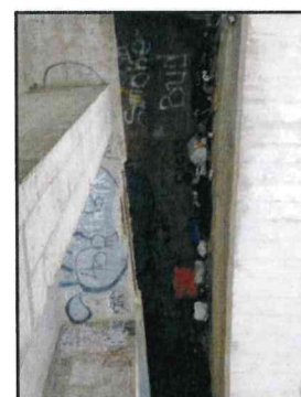
12 : Spall Repair on Span 10 exterior Girder. (North Girder Shown, South Girder similar)
