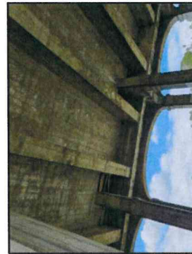
14 : Spall Repair on Span 12 and 13 Exterior Girder. (North Girder Shown, South Girder similar)
