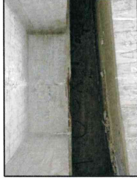
⑩ : Spall repair in Span 9 Exterior Girder (North Girder Shown, South Girder similar)
