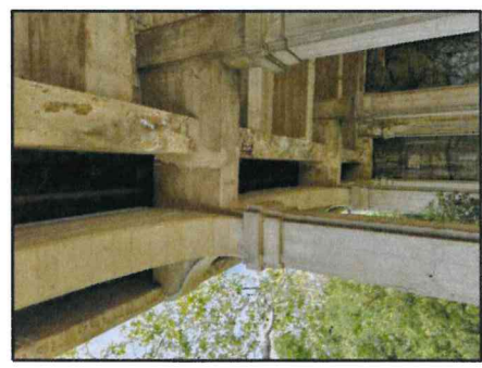
④: Span 2, 3, 4 spalled exterior girder (south girder shown, north girder similar)
