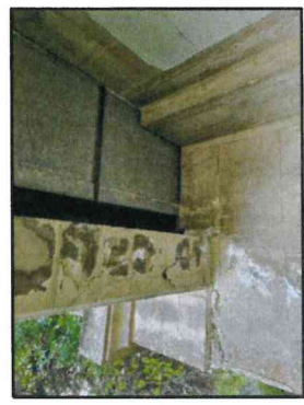
19 : Spall Repair on north exterior girder, (North Girder Shown, South Girder Similar)
