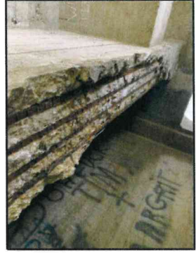
⑧ : Spall Repair on Span 7 exterior Girder. (South Girder Shown, North Girder Similar)
