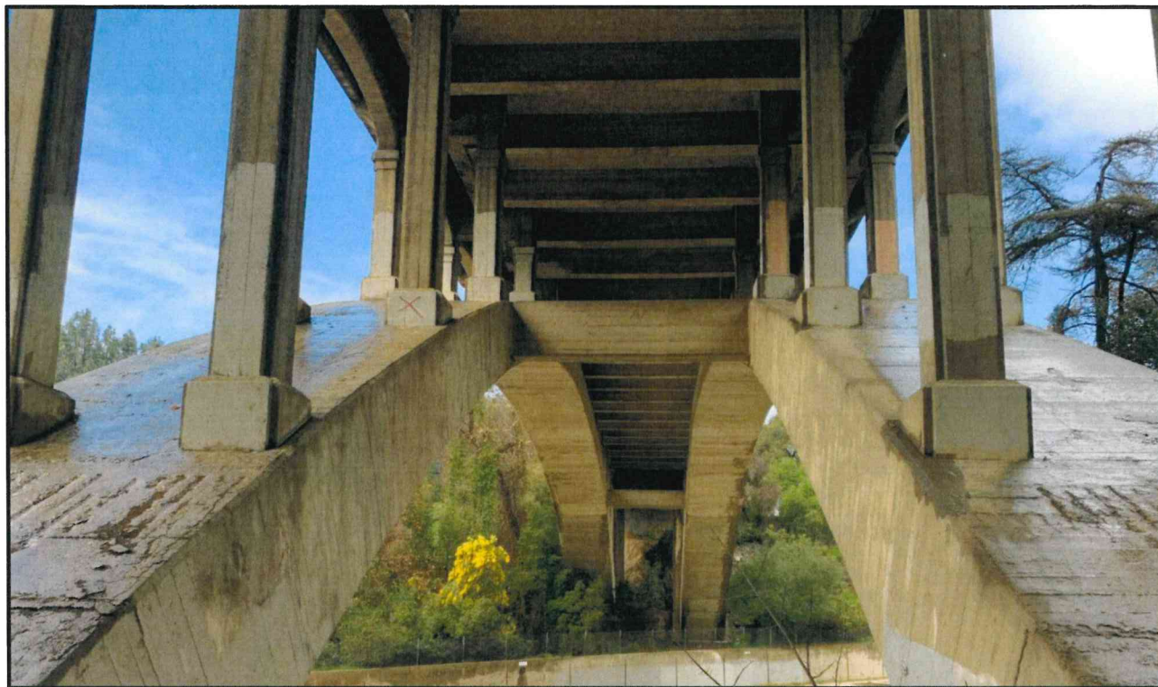
The Holly Street Bridge spandrel columns view facing northwest. Source: Dokken Engineering (2019).
