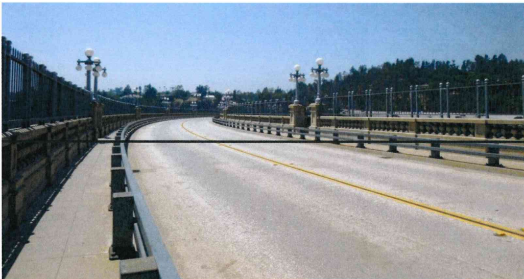
Image showing a view of the Colorado Street Bridge crash barrier. A similar barrier is proposed to be added to the Holly Street Bridge
