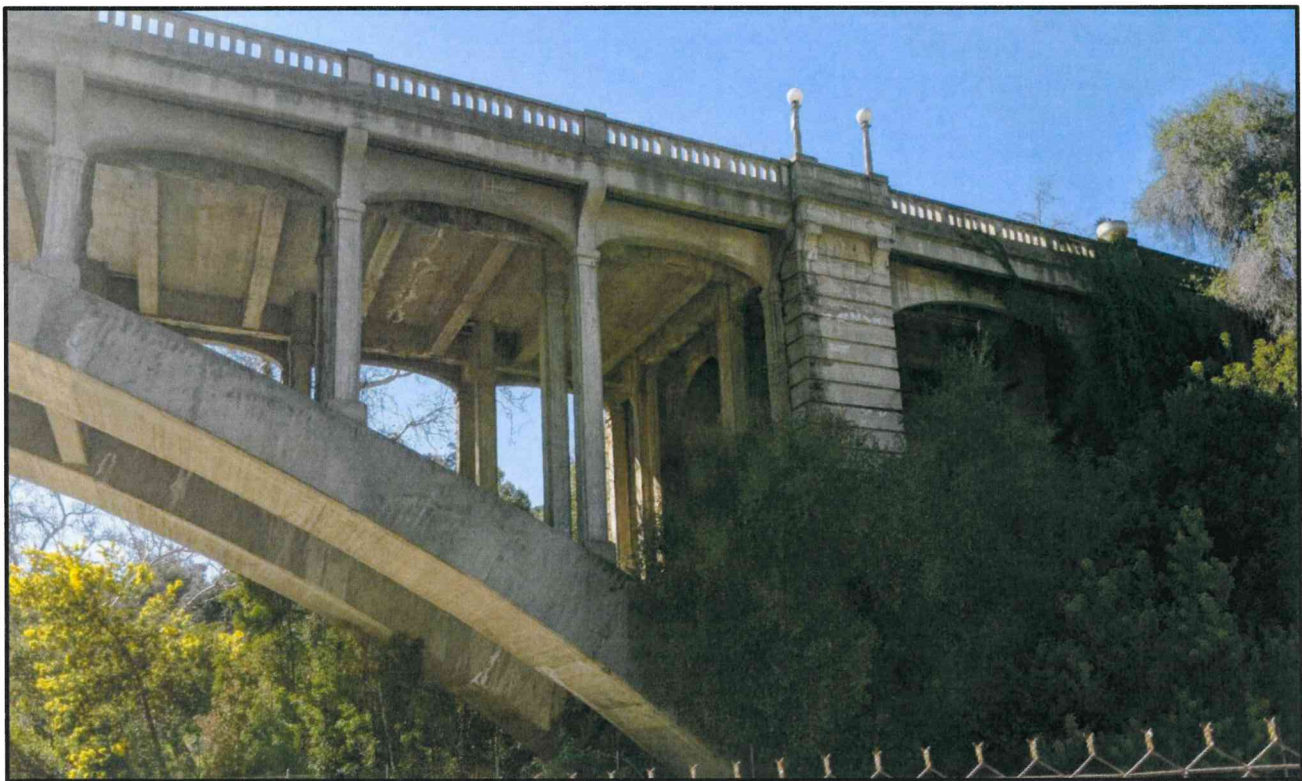
The Holly Street Bridge spandrel columns, view facing south. Source: Dokken Engineering (2020).
