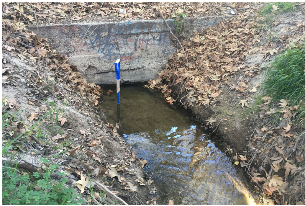
February 10, 2022. View of wetland sampling point 1, near outlet structure at upstream end of San Pascual Basin area. Note that the outlet structure in background is nearly completely filled with sediment.
