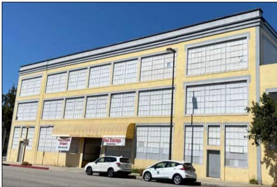
Figure 9: East elevation of the daylight factory on South Raymond Avenue, showing expansive window bays (Reyes 2021).
