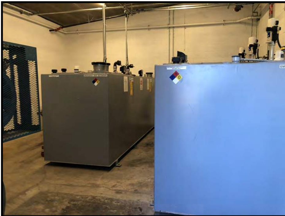
View of the aboveground tanks for used antifreeze and new motor oil near the service area on the eastern portion of the subject property.
