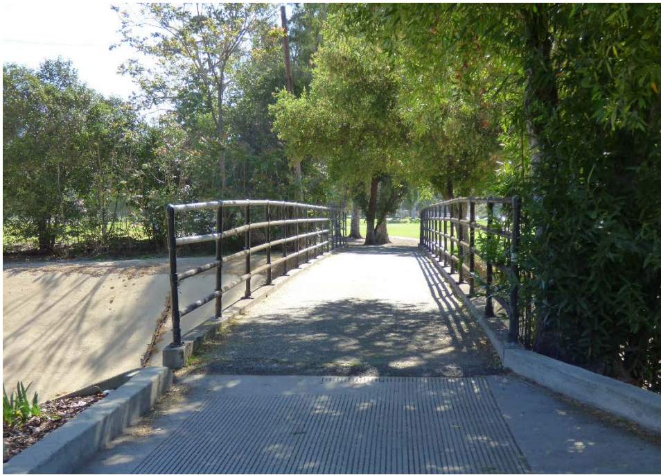
Detail of concrete bridge over Arroyo Seco Channel looking east. Historic Resources Group, 2021.
