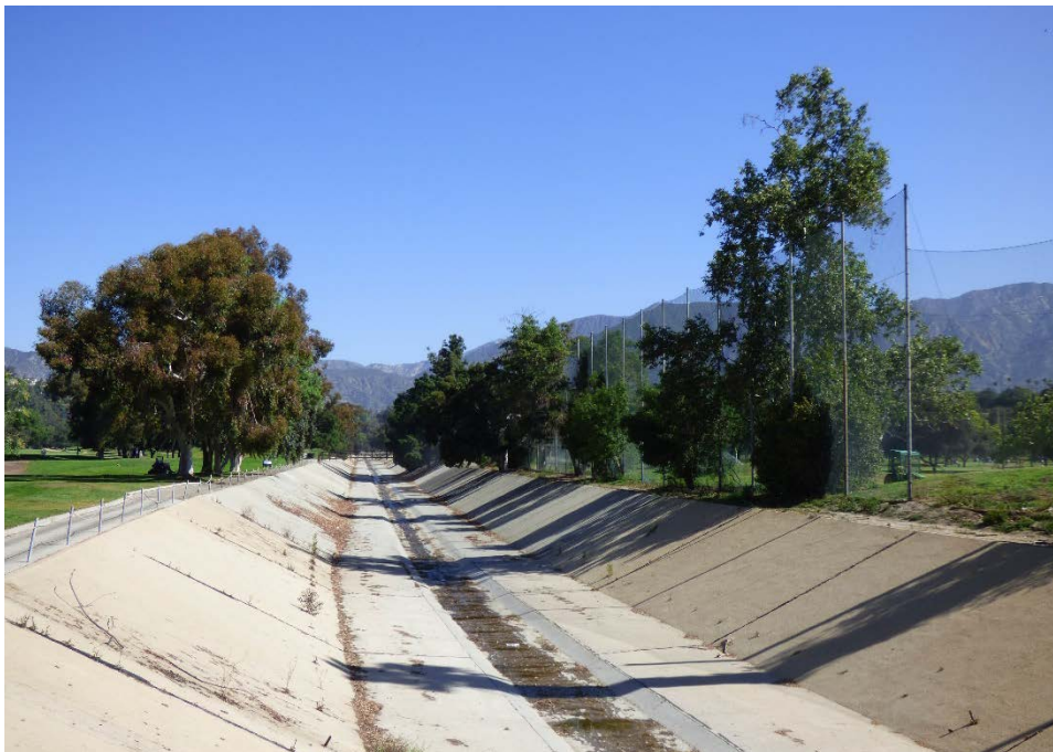
View of Arroyo Seco Channel immediately west of the driving range looking north. Historic Resources Group, 2021.
