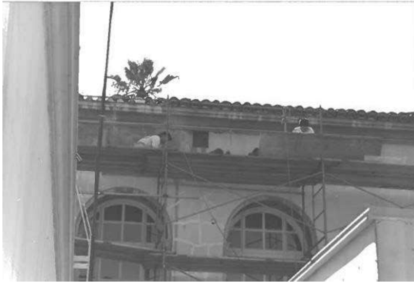
Photos of damage post 1991 Sierra Madre Earthquake (5.6 magnitude)
