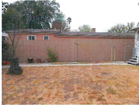
Figure 24: Concrete paving along remainder of rear yard and lawn area. Looking west.
