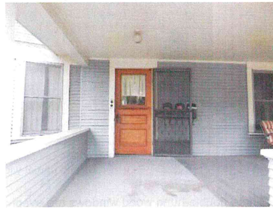
Figure 9: Front door recessed beneath porch Light fixture at porch ceiling. View looking south.
