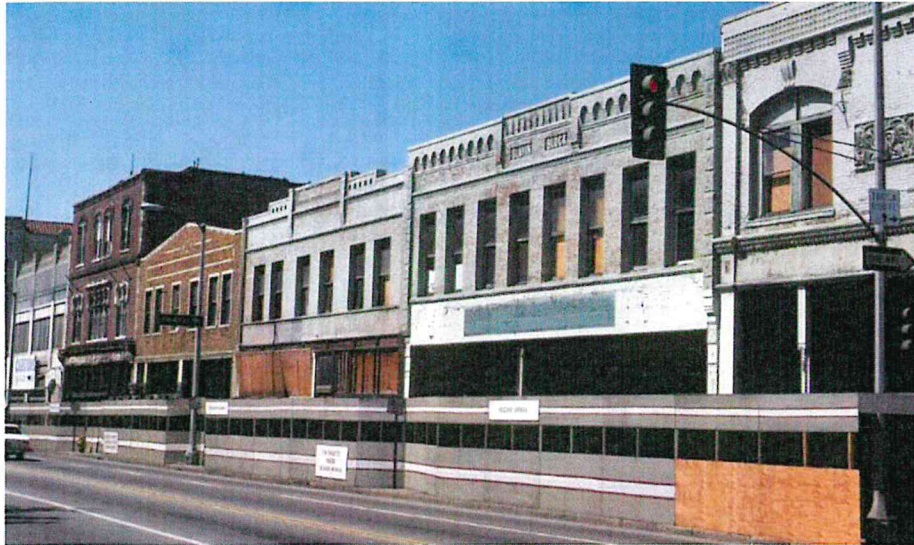
Figure 35: Commercial properties along Fair Oaks Avenue in the process of rehabilitation, ca. 1980. Source: OldPasadena.org
