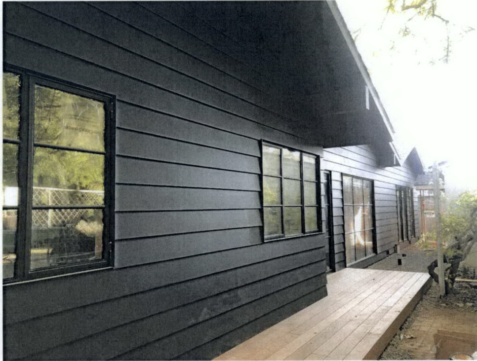
Figure 8. Southwest Façade, 801 S. San Rafael Avenue (view southeast) SOURCE: Sapphos Environmental, Inc., 2021
