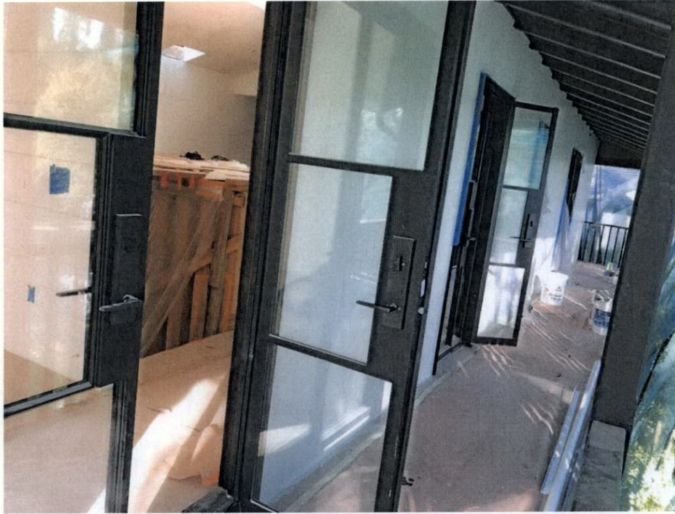
Figure 5. Second-Story Primary Façade, 801 S. San Rafael Avenue (view west) SOURCE: Sapphos Environmental, Inc., 2021
