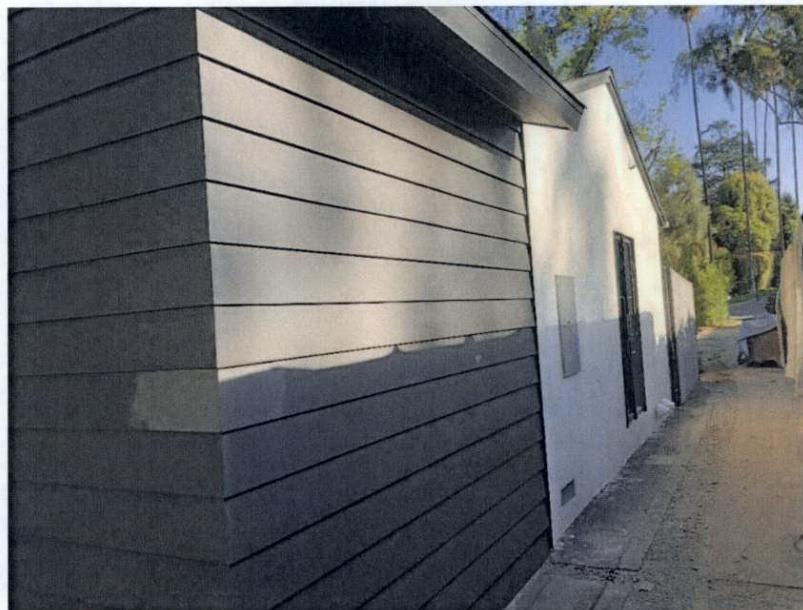
Southeast Façade, 801 S. San Rafael Avenue (view north) SOURCE: Sapphos Environmental, Inc., 2021
