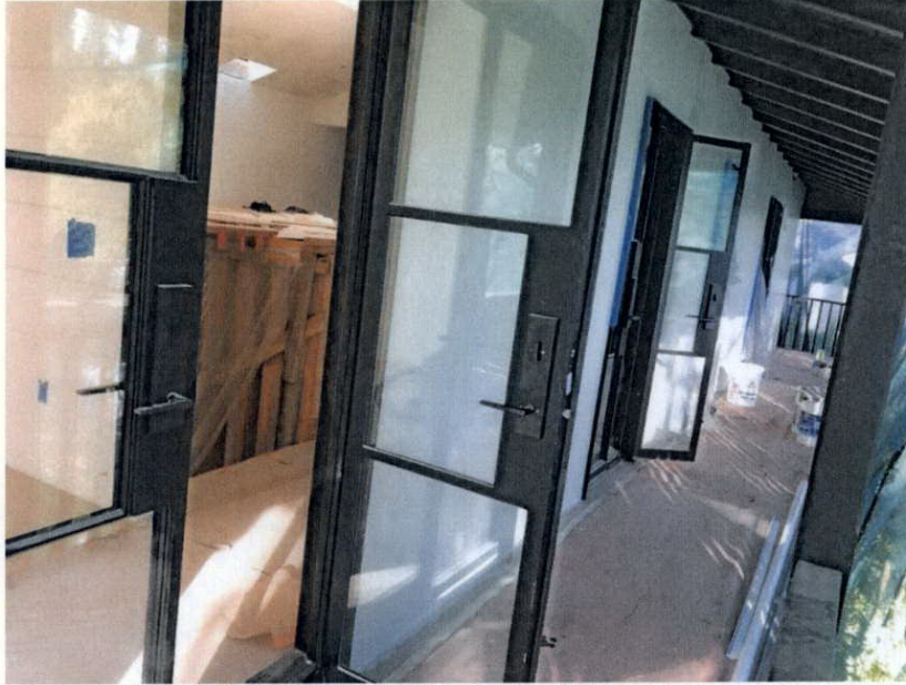
Second-Story Primary Façade, 801 S. San Rafael Avenue (view west) SOURCE: Sapphos Environmental, Inc., 2021
