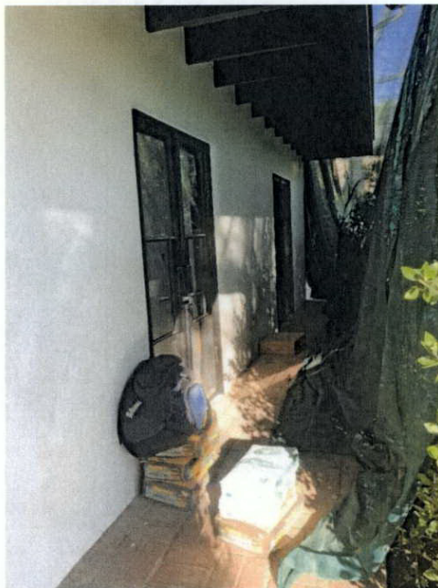
First-Story Primary Façade, 801 S. San Rafael Avenue (view west) SOURCE: Sapphos Environmental, Inc., 2021
