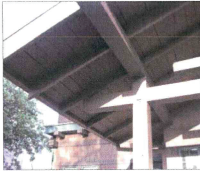
D. Exposed rafter tails
