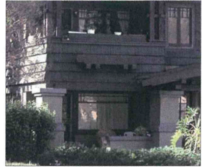
C. Painted shakes above painted plaster
