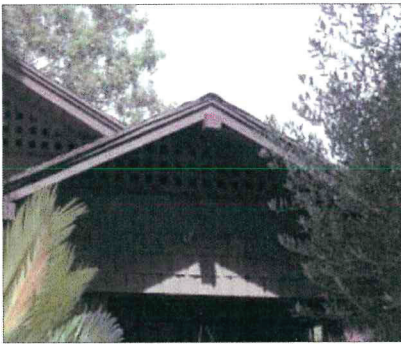
D. Attic vents placed at gable ends
