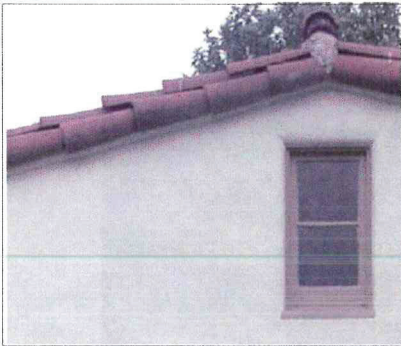
D. Tile roof without eaves
