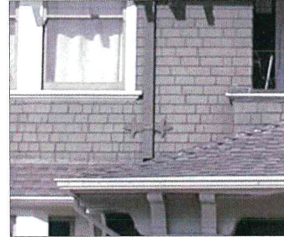
F. Downspout attached to wall with decorative strap
