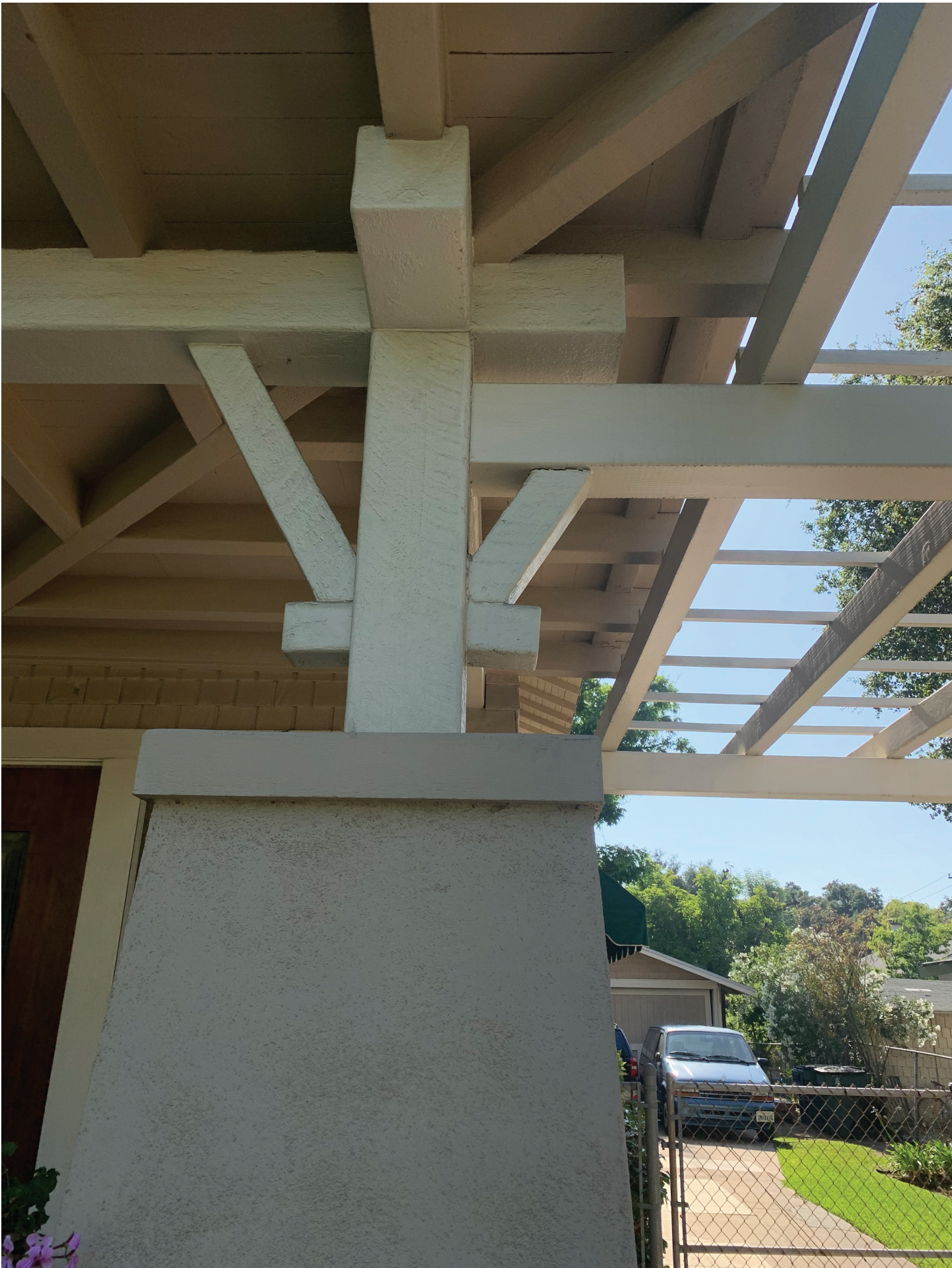
1500 N. LOS ROBLES AVE: FRONT PORCH PIER AND POST DETAIL WITH PORTE COCHERE TO THE RIGHT
