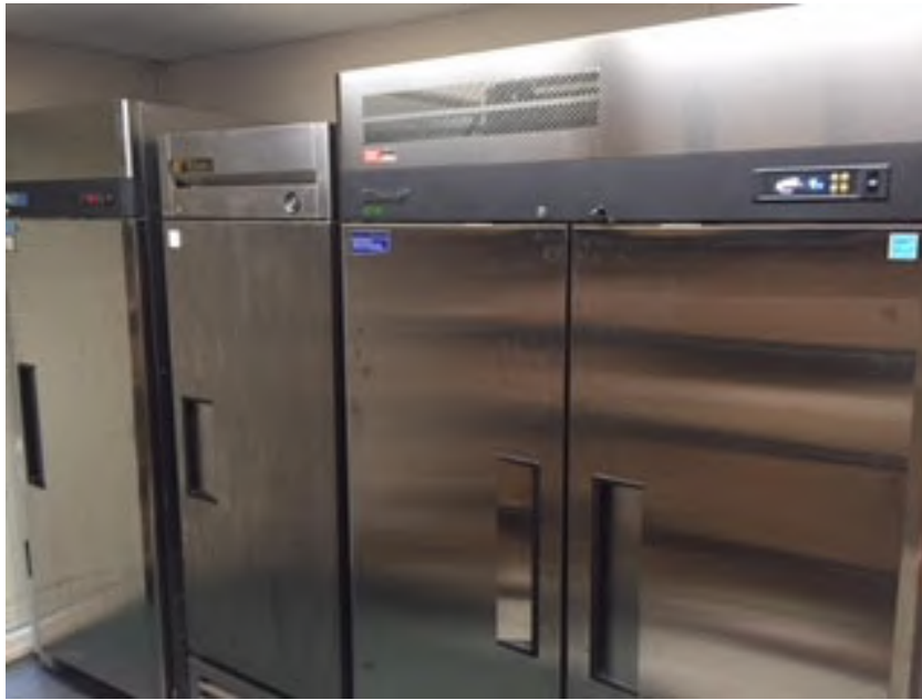
View of the refrigerators.
