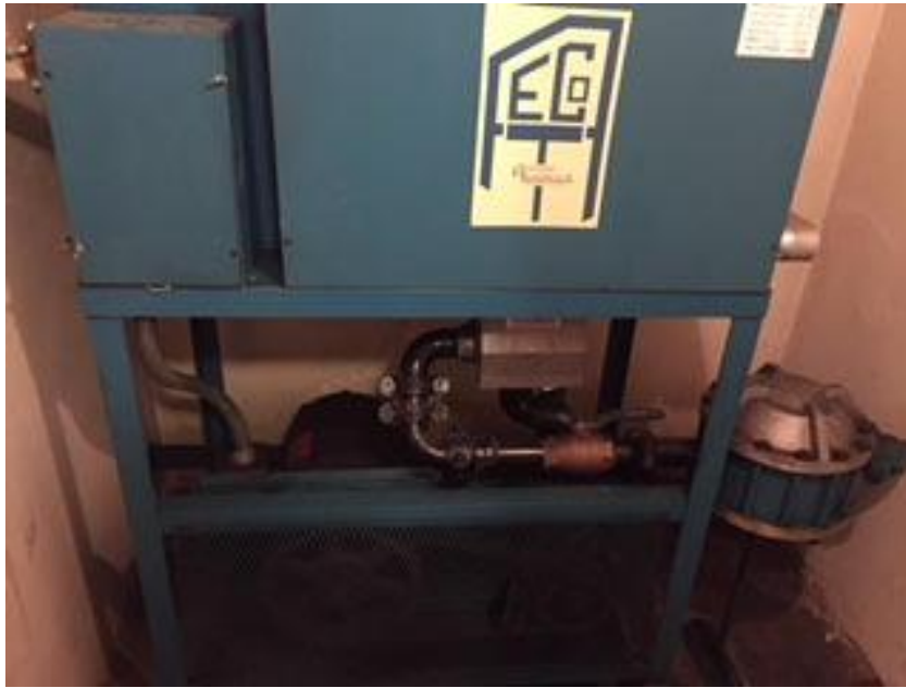
View of the elevator equipment.
