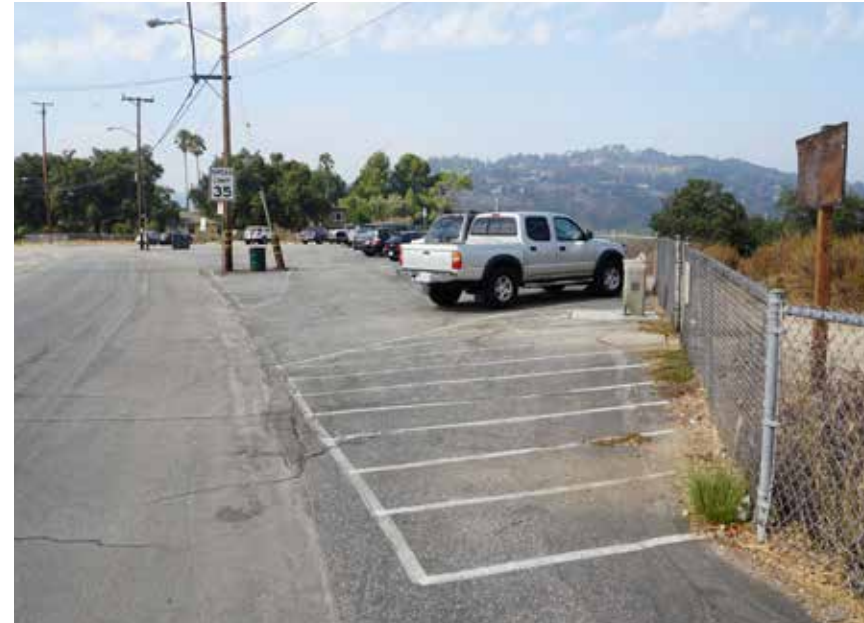
Existing parking at Hahamongna East, asphalt condition
