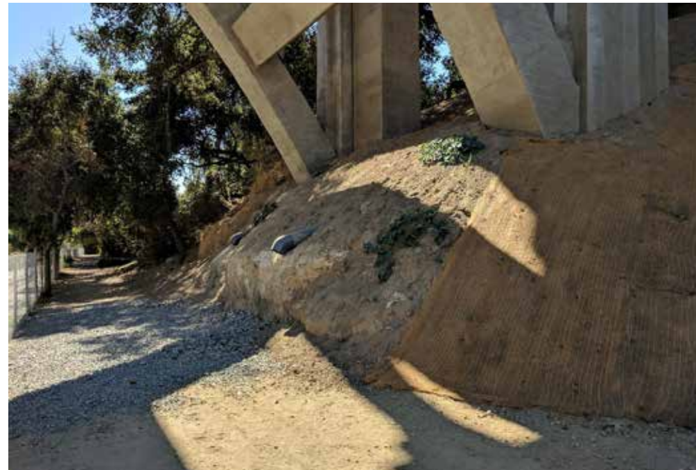
Trail Erosion / Surface Water Run-on
