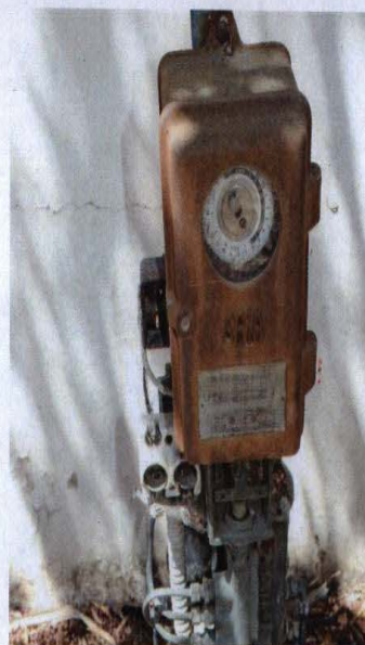
The original (?) irrigation controls for the front yard.
