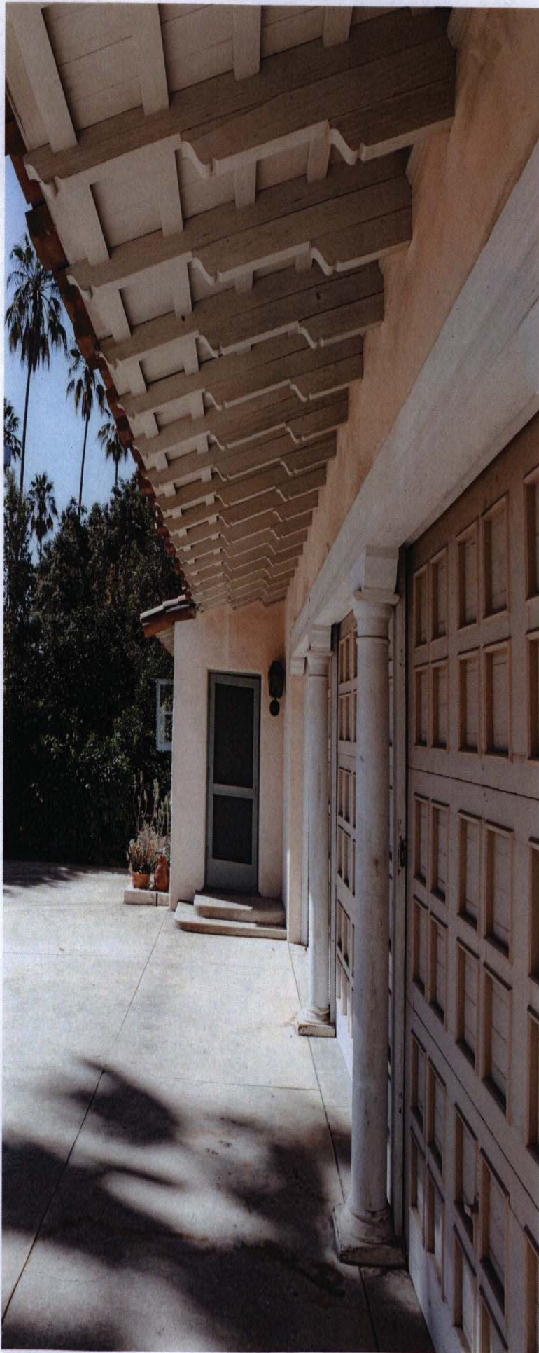
Looking south at the front door of the Chauffeur's Quarters. Not the detail in the rafter tails of the roof.
