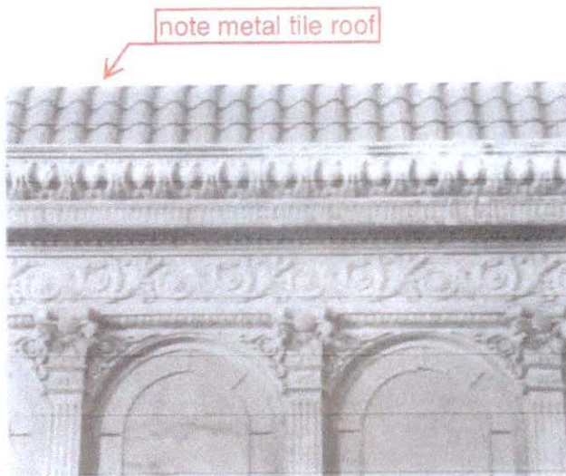
Figure 23. Pressed Copper Sheet Metal Cornice, Frieze, and Pilasters; Conservatory of the Christian Heurich Mansion, 1307 New Hampshire Avenue, NW, Washington, D.C., 1902; Appleton Clark, architect. The copper work was assembled from many pieces of sheet copper pressed with low relief designs. (Jack E. Boucher. NAER)
