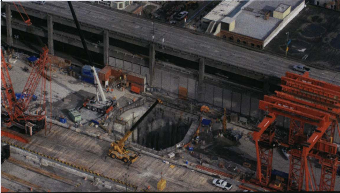
Feb. 13, 2015 - Aerial photo of the 120-foot-deep pit crews will use to access and repair Bertha, the SR 99 tunneling machine. Washington State Dept of Transportation
