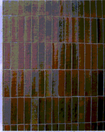
WALL TILE | The materialistic quality of this element helps support the character defining features of the architecture. Used as a main exterior wall 'in fill' finish in limited applications to define mass at the corners of the building. Note the variance in tone, size and pattern of the tiles.
