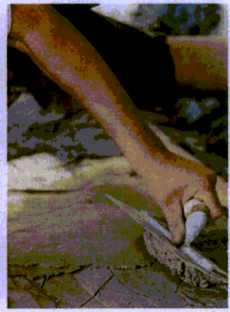
POLISHED COLORED CONCRETE + SMOOTH PLASTER | This can be used as a main tectonic and materialistic unifying design element. Aside from polished colored concrete, other suitable substitutes are smooth plaster or metal panels in a similar color. Can be a main element or can also be used in limited applications in conjunction with patterned tactile in fill wall panels or glazing. Painted and well articulated structural steel can imply a similar character.
