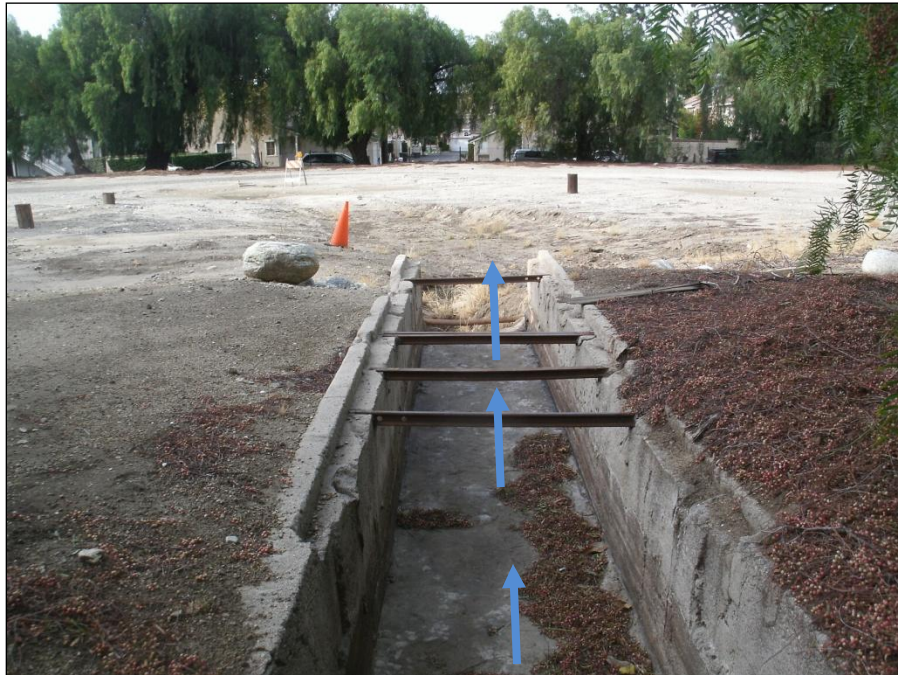
Photo 3: Picture taken facing west. The picture shows the culvert located in the east portion of the proposed staging area. The blue arrows indicate the direction of water flow.
