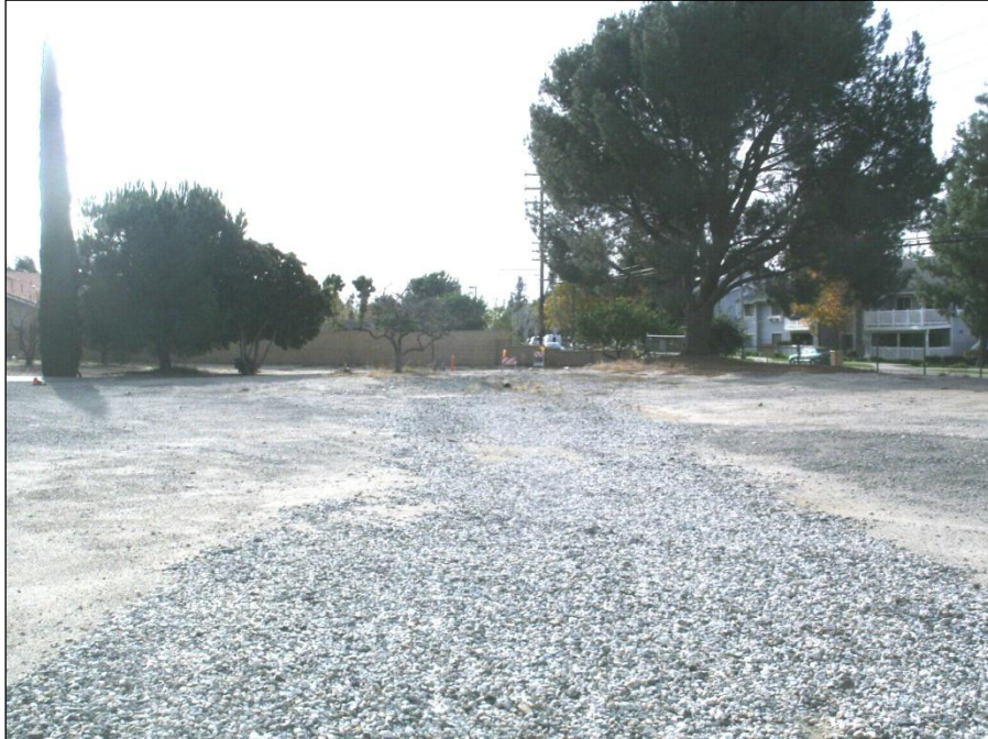
Photo 5: This photo was taken facing south from the center of the proposed staging area. The photo shows the path of water that is diverted through a 1 ft. plastic pipe into the catch basin.
