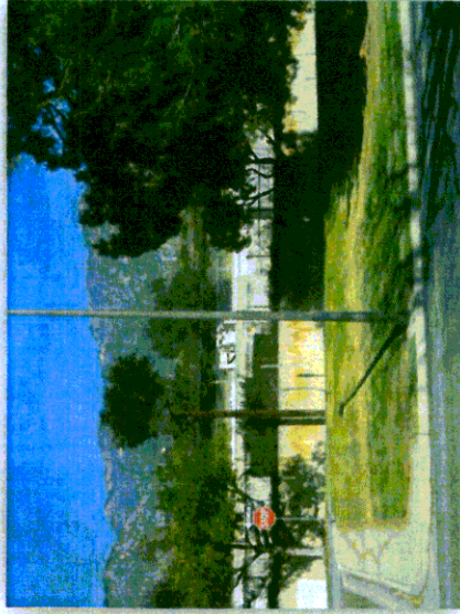
North-Facing View of PWP Equipment at Jones Reservoir Adjacent to Centralized Disinfection Facility Site
