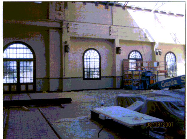
Turbine Hall tile and lamps
