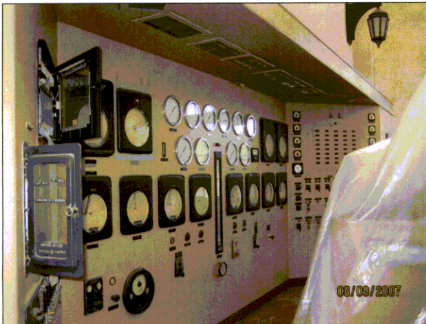
Turbine Hall control panel detail
