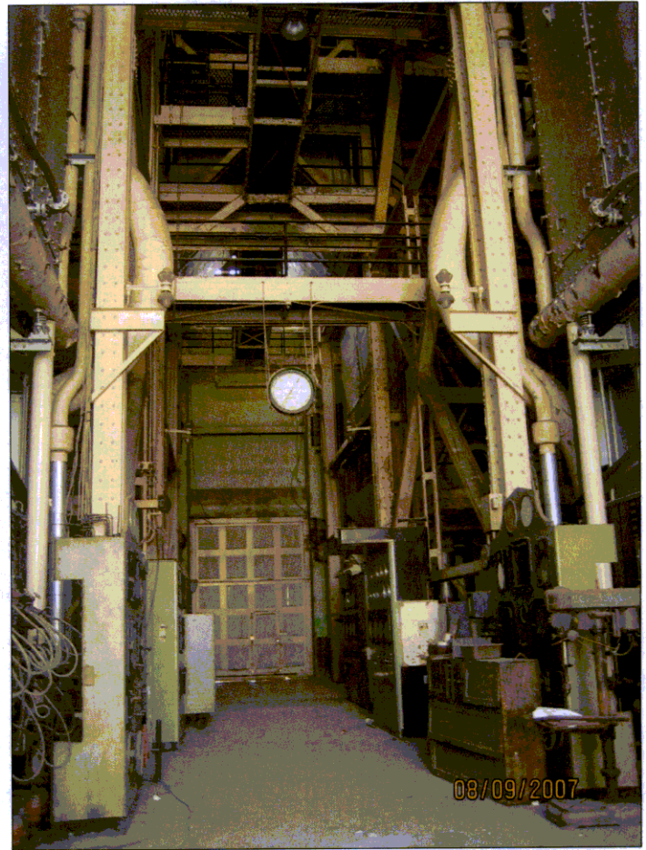
Boiler Room hallway (west end - current)
