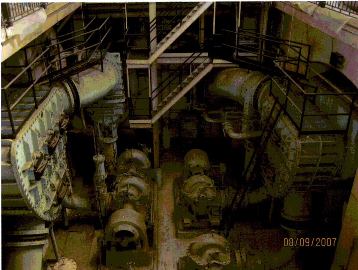
Mechanical well/condenser units (current)
