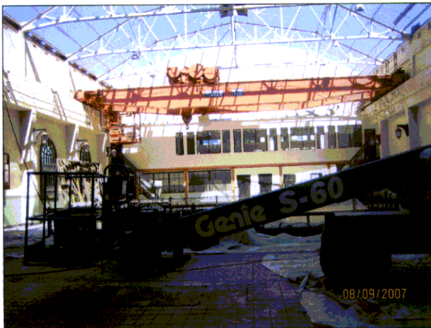
Easterly portion of Turbine hall
