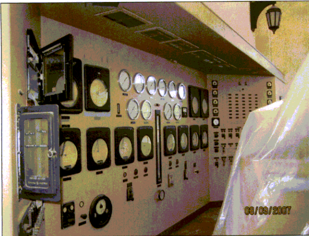
Turbine Hall control panel detail
