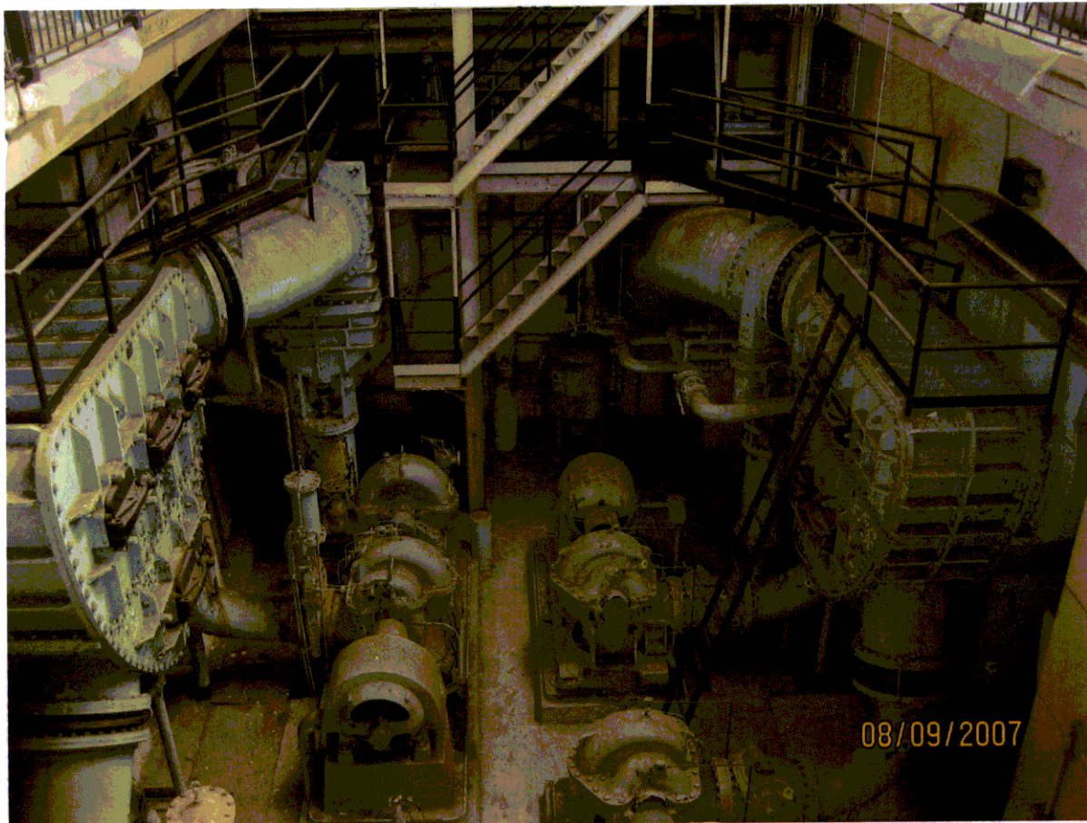
Mechanical well/condenser units (current)
