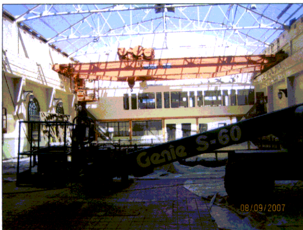
Easterly portion of Turbine hall
