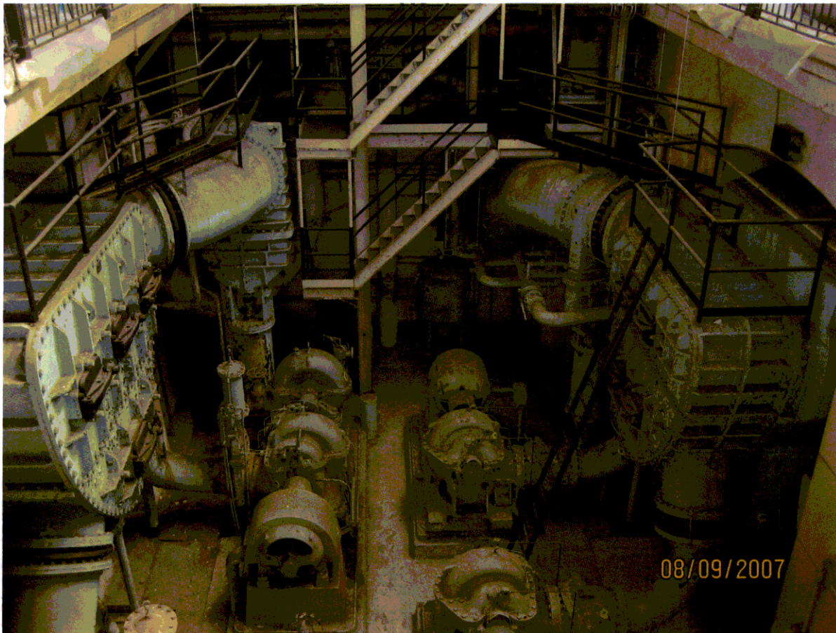
Mechanical well/condenser units (current)
