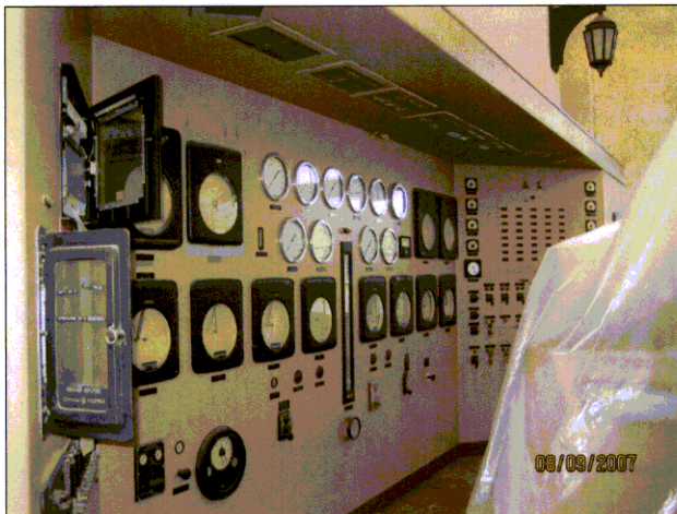
Turbine Hall control panel detail
