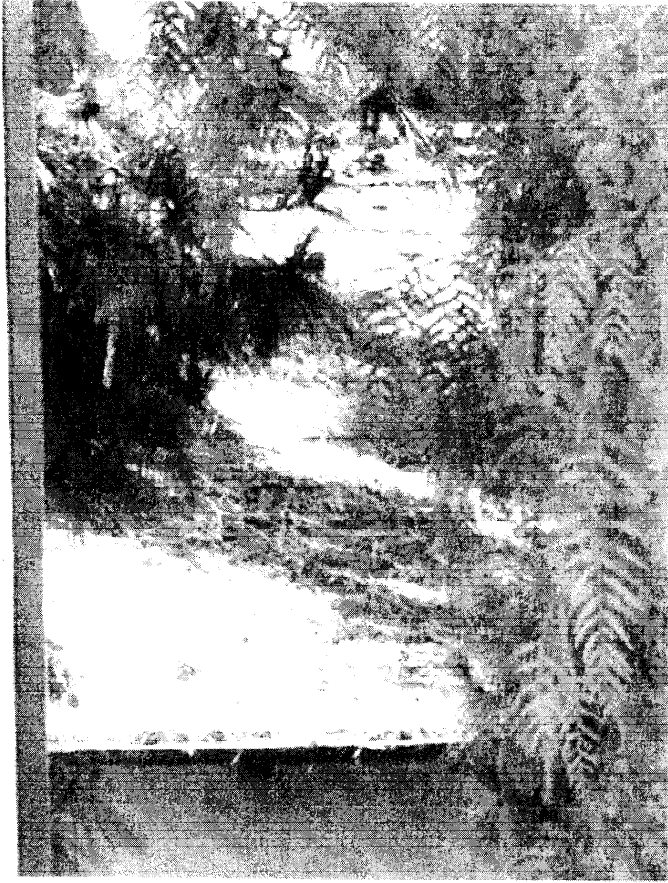
Figure 9- Close-up from Figure 8 showing significant deposition of highly flammable and dry debris on unpermitted wood roof.
