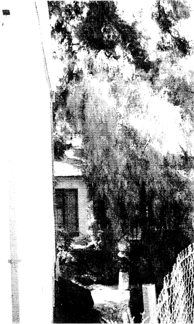
Figure 8- Structures with unpermitted wood roofs immediately adjacent flammable vegetation. (See also Figure 9)
