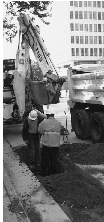
Implementation of the Water System Master Plan is well underway, with more than 12 miles of aging pipeline already replaced.
