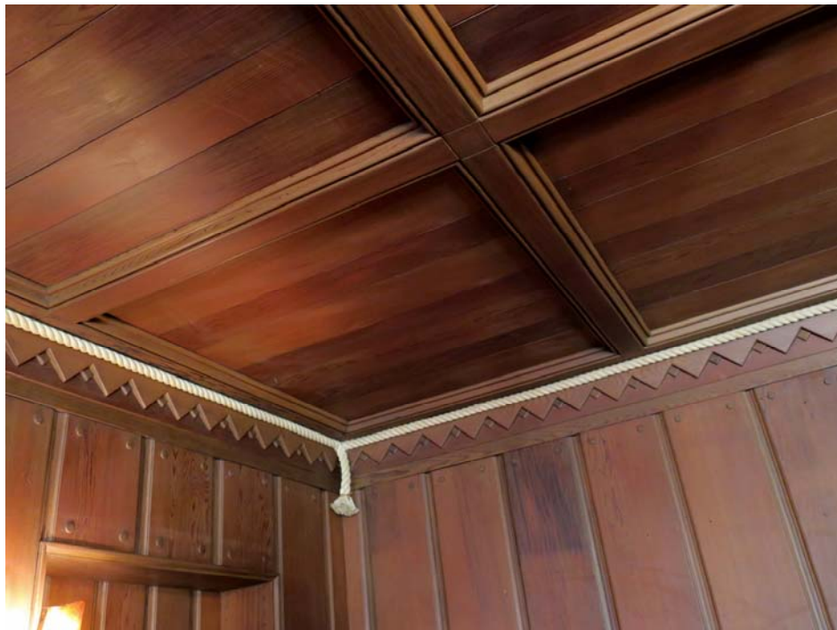
Detail of coffered wood ceiling, wood-and-rope molding, and paneled wood walls in den.
