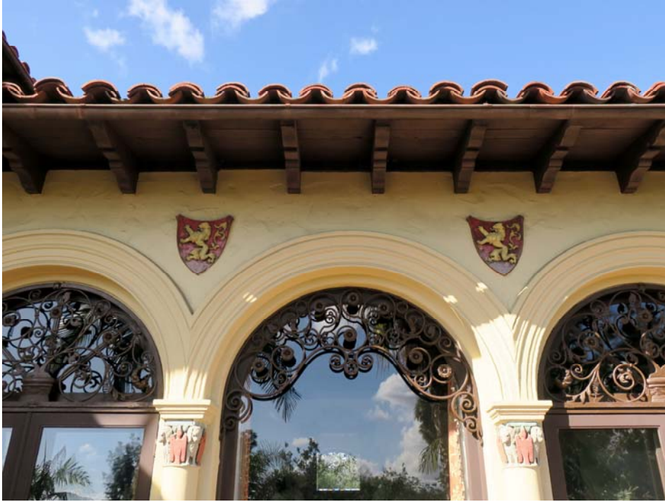
Detail of decorative surrounds, engaged columns, iron grilles, and escutcheons on rear elevation, view west.
