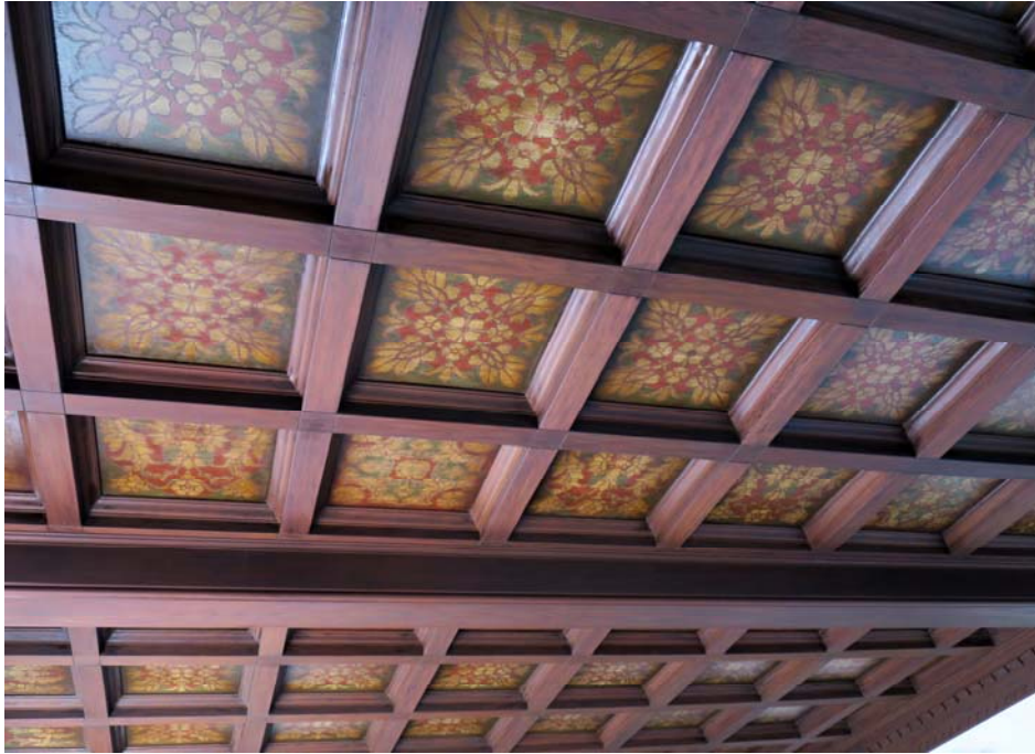
Detail of offered wood ceiling in living room, with hand stenciled details and denticulated molding
