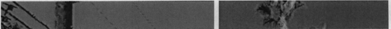
Small cell (circled in red) on a pole-to-pole strand in Torrance, California; at right, a small cell mounted onto a pre-existing light standard. Photographs courtesy of the City of Pasadena
