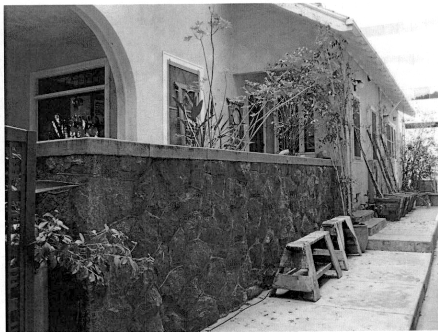
Figure 6. Looking northeast at the quartz stone wall, located at the southwest corner of the building. Note the missing Doric columns and wooden pergola structure.
