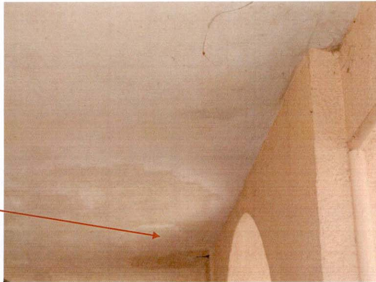
Figure 1: Damage to Soffit at Porch Entry (Looking South)
