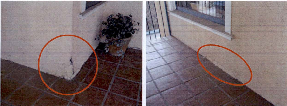
Figures 6 & 7: Damage at Porch (Looking East)
