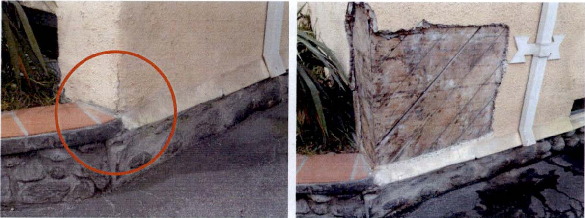
Figures 14 & 15: Crack at Foundation Corner (Looking Southwest)
