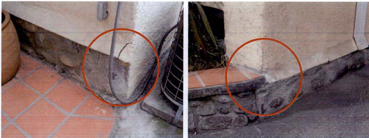
Figures 12 & 13: Cracks at Foundation Corners (Looking Northwest & Southwest)
