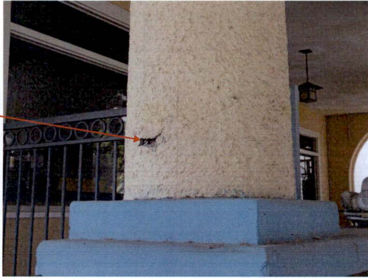
Figure 3: Cracks at Entry Column (Looking South)
