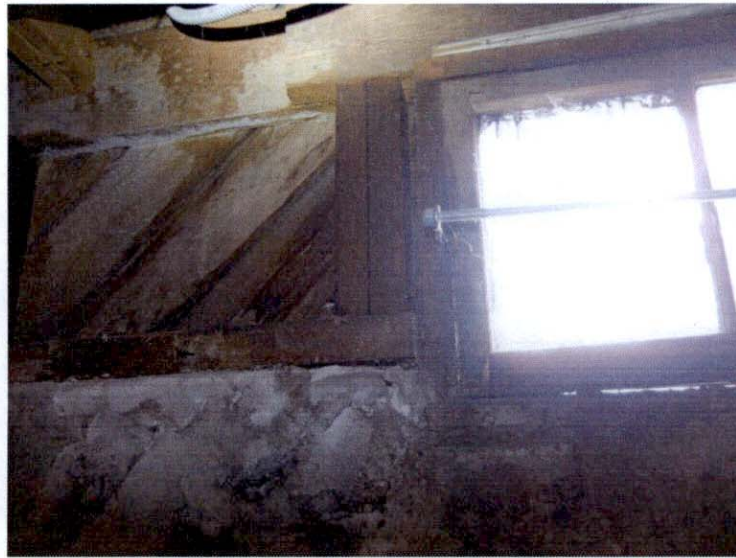
Figure 8: Moisture at Foundation (Looking North)
