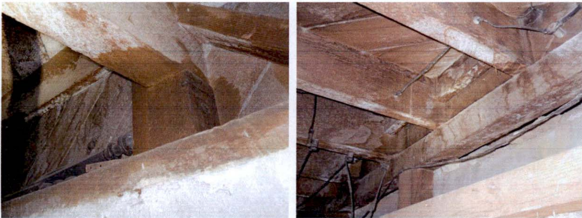
Figures 9 & 10: Moisture at Foundation (Looking West)
