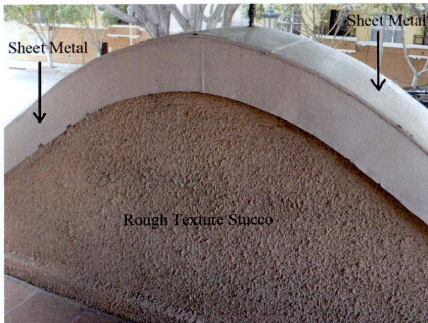
Figure 2. Looking west, within upper porch, at the sheet metal coping over parapet with a rough texture stucco wall surface.
