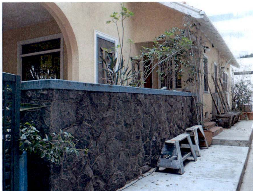
Figure 6. Looking northeast at the quartz stone wall, located at the southwest corner of the building. Note the missing Doric columns and wooden pergola structure.
