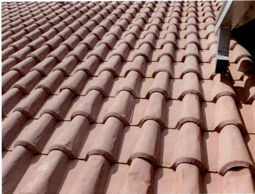
Figure 1. Looking east at the sheet metal roofing imitating a red clay tile roof, primary west elevation.
