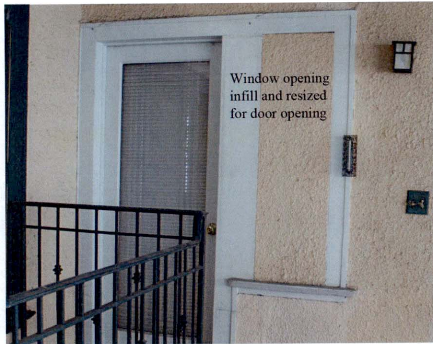
Figure 9. Looking north, south elevation of rear upper story, window opening infill and resized for door opening; 1994 alteration permit.
