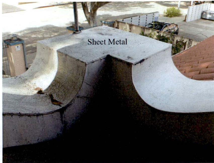
Figure 3. Looking northwest at the sheet metal coping imitating a Mission Revival stucco feature.
