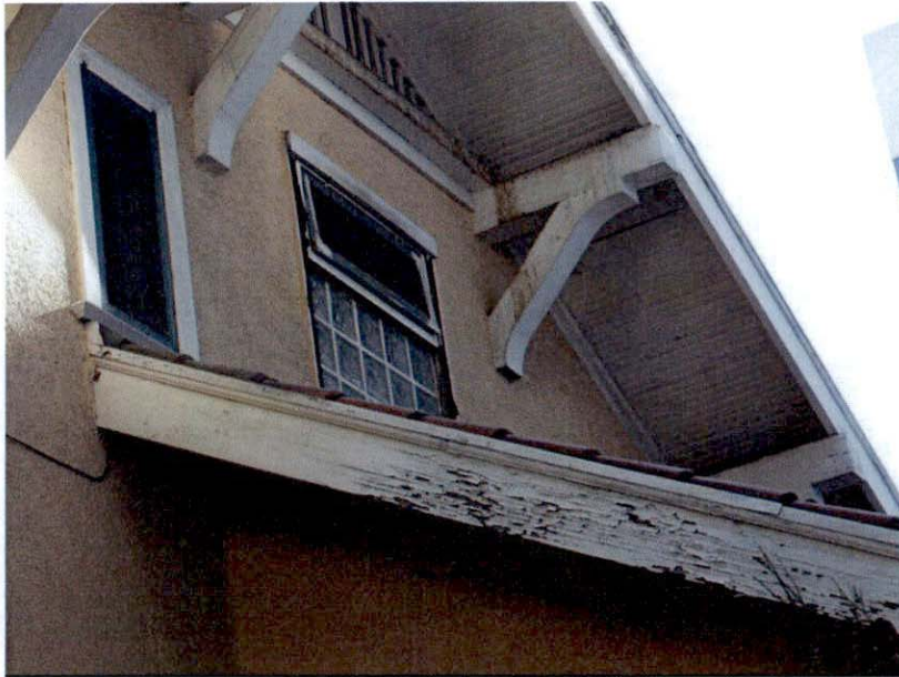
Figure 7. Looking northeast within the upper gable end showing an aluminum hopper window with glass-block window units.
