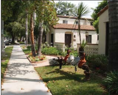
⚠ A back flow preventer that is completely visible from the street and sidewalk
