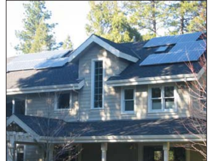
⚠ These solar panels are randomly and haphazardly placed.
