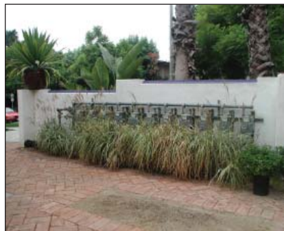
Gas meters screened by native plantings.
