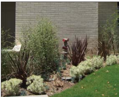
A back flow preventer that is located immediately adjacent to the building and is screened from the view of the sidewalk and street by shrubs.
