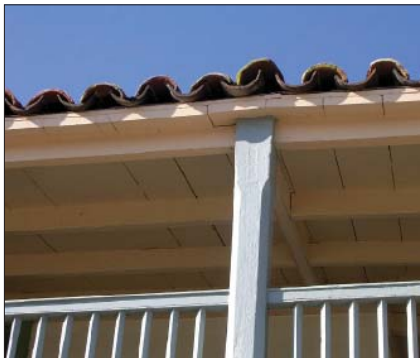
D. Clay tile roof without eaves
