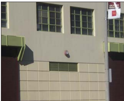
This vent grille aligns and relates to the adjacent gridded wall pattern.
