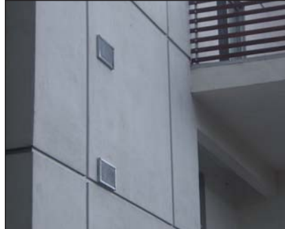
⚠ Vents introduced into a building late in the design process appear to be an afterthought.
