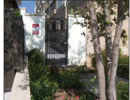
Gas meters that are screened from the view of the sidewalk and street by a wall and gate. The subterranean electrical transformer vault is screened by shrubs.
