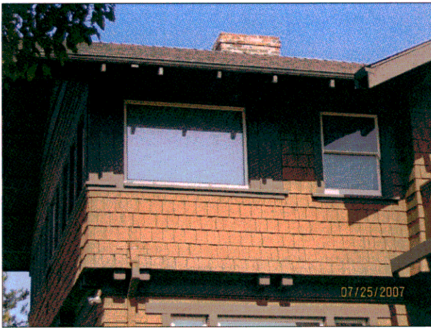
Non-original window – Lake elevation
