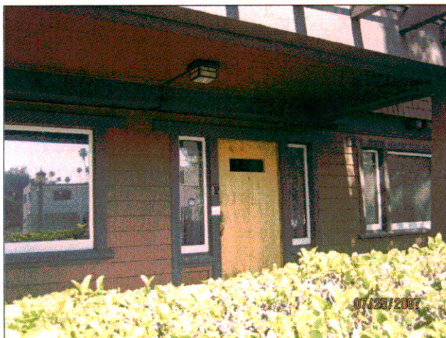
Non-original front door
